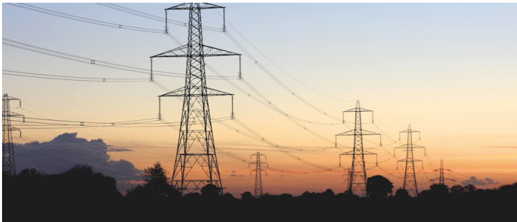
Figure: AC power lines.
