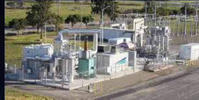
Fuel Cell Power
